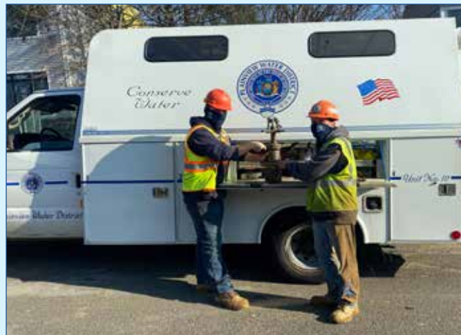
Plainview Water District Water Servicers John Curro (Left) and Frank Caraturo (right) preparing a tapping machine as part of a new water service installation.
